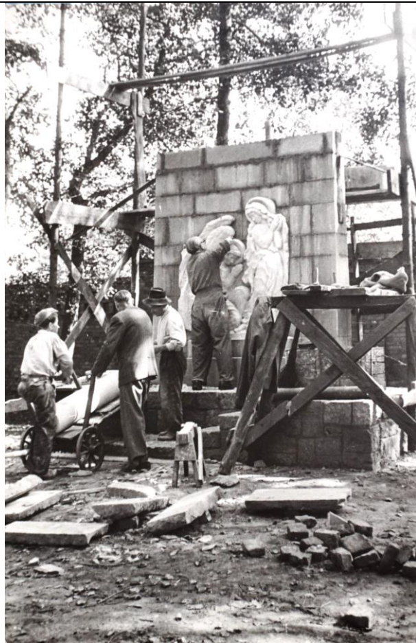
46. Karol Muszkiet and workers during the construction of the Annunciation chapel, 1957. The Archives of the Franciscan Friars of the Assumption of the Blessed Virgin Mary Province.
